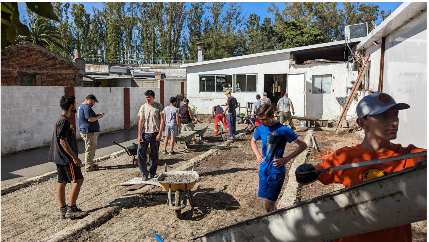
A lot of our men helped pour the foundation for the new fellowship hall which we will build, Lord-willing, in January.
