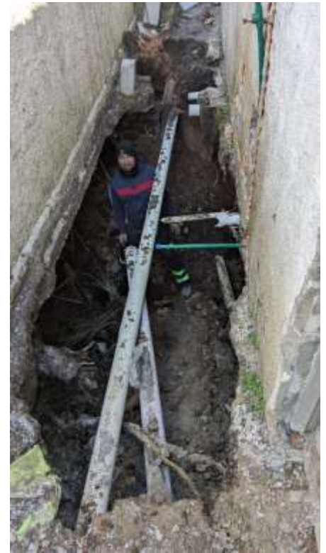
Surprise sink hole!
